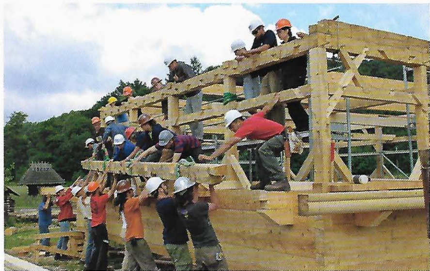
A team of students and professional craftsmen from the Timber Framers' Guild assemble beams for the synagogue roof structure.
